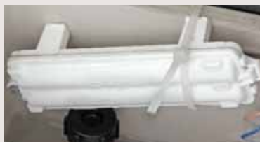
Close up of open cistern showing battery operated power unit.
