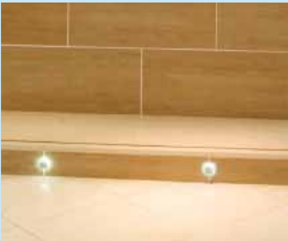
Wall to floor showing 60cm x 30cm Roma gloss ivory wall and beige matt floor tiles.
